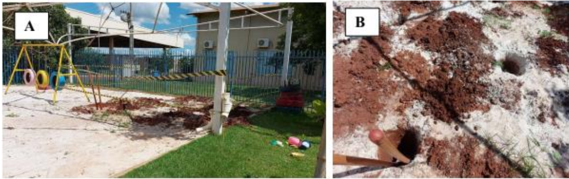
Figure 8. (A) View of the oca space with the openings of the holes for the foundation. (B) Detail of the openings for fixing the pillars.
